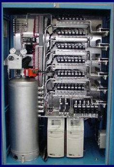
Hazardous Gas Monitoring
