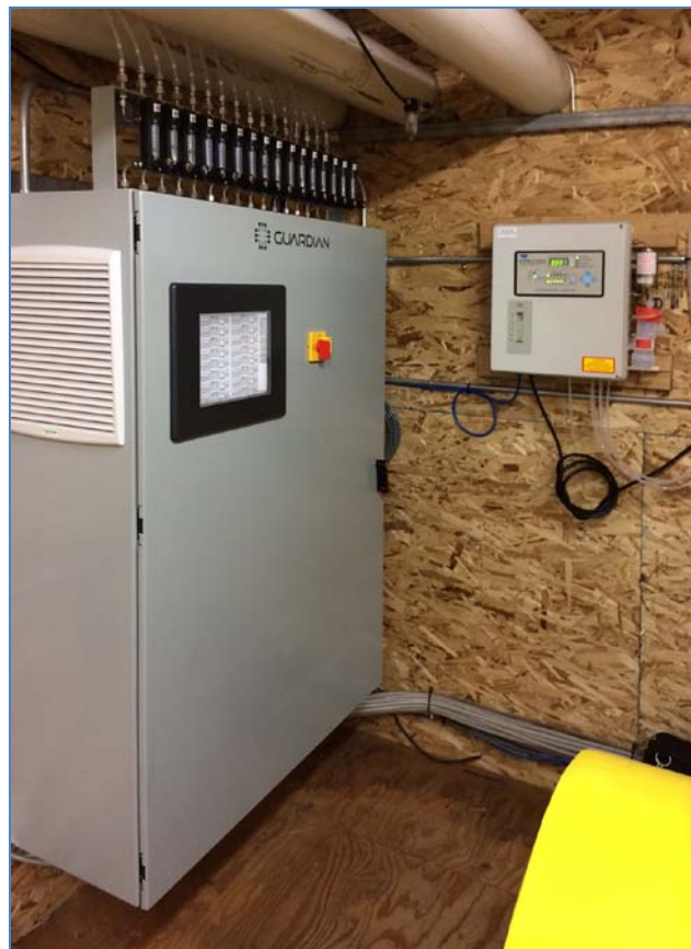
Sixteen manifold Guardian Ensure Smart™ ozone system installed at a controlled atmosphere storage facility in Washington.
